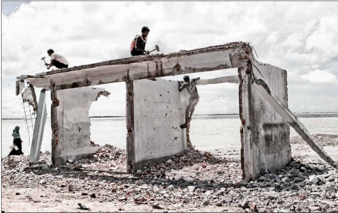
Figure 5. A building structure is being removed as the Padma River gets closer. Location: Padma River, Mawa, Munshigonj, Bangladesh Date: 20 September 2013
