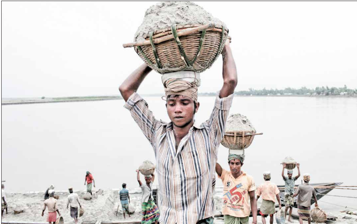
Figure 21. Workers bring sand to dump at the river bank to protect their villages from flooding. Location: Jamuna River, Islampur, Jamalpur, Bangladesh Date: 5 October 2013
