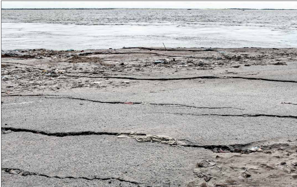
Figure 4. Roads, markets and houses are swallowed up by the Padma River during the flood. Location: Padma River, Mawa, Munshigonj, Bangladesh Date: 20 September 2013
